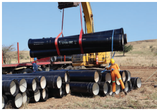
Arrival of Ductile pipe for Ntambanana Water Supply and Pump Station Construction
