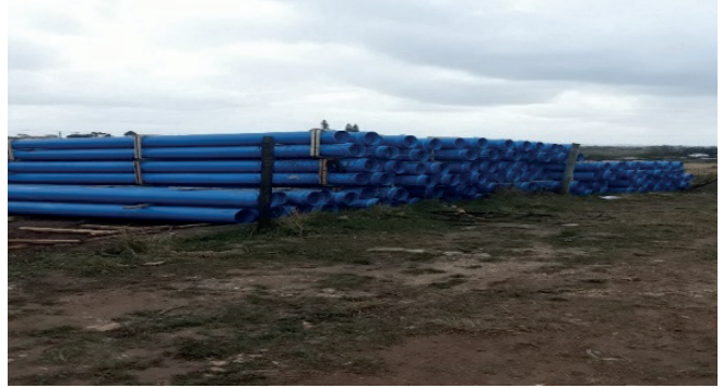
315mm pipes ready to lay at Mhlana Somopho Somopho bulk water pipeline project/ King Cetshwayo District Municipality
